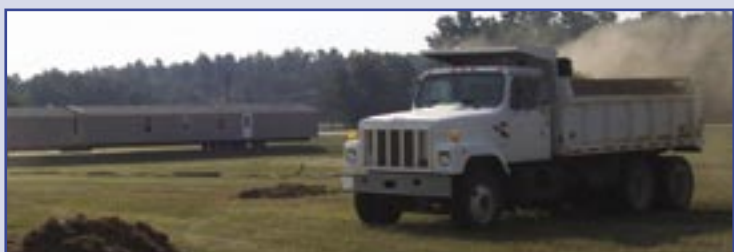
Texarkana, TX September 7, 2005 - Day and Zimmermann, Inc. workers at Lone Star Army Ammunition Plant prepare the grounds to receive an estimated 25,000 mobile homes and recreational vehicles which will be sent throughout Texas and Louisiana as temporary housing for victims of Hurricane Katrina. In the background are two of several mobile homes already at the ammunition plant. Day and Zimmermann, Inc. is the contract operator of LSAAP located in Texarkana. (U.S. Army photo by Mark Hughes)
