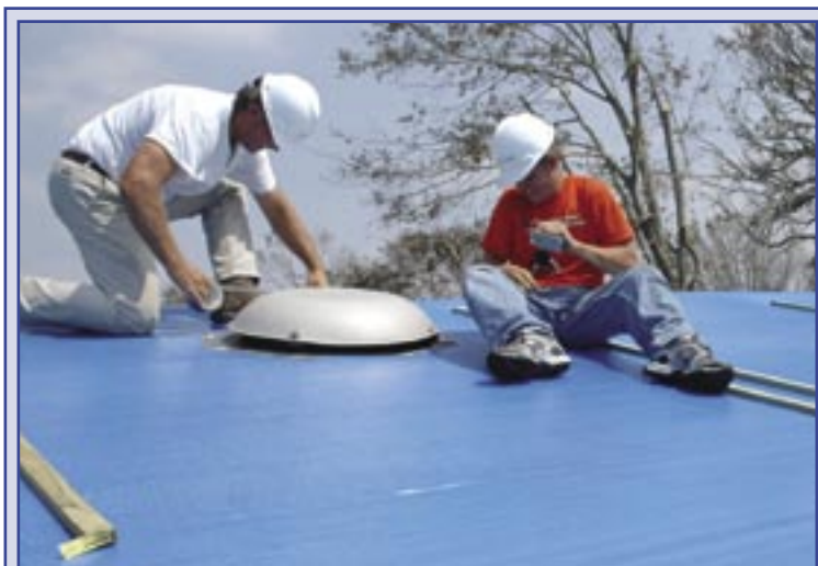
Biloxi, MS, September 12, 2005 - A construction crew from San Antonio, TX installs tarps as part of the USACE Blue Roof program. Hurricane Katrina damaged countless roofs throughout Mississippi.
